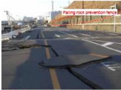
Falling rock prevention fence One side of the road on the westside was cracked and subsided in parallel with road. West side was accessible. Photo taken 3/17
