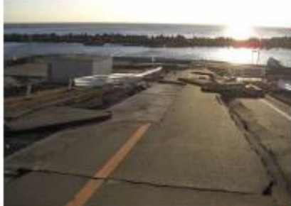
Reinforcement work was conducted on this road, but cracks and subsidence was found on both sides of the road which were not reinforced. Photo taken 3/17
