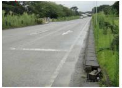
No particular abnormality found with straight road from main gate. Photo taken 8/26
