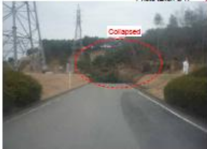
Though not a priority emergency route, the slope failed and the road was blocked and impassable. Photo taken 3/20
